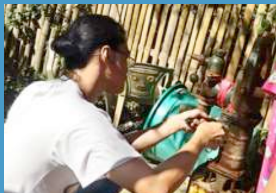
Fixing the water pump at the Mampang Ministry Center; since this is just a few meters from the seashore, water is a bit salty and sandy.
